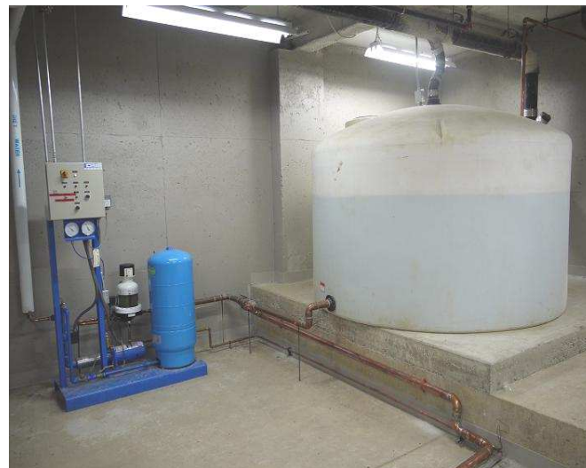
Indoor rainwater storage tank located in the basement
