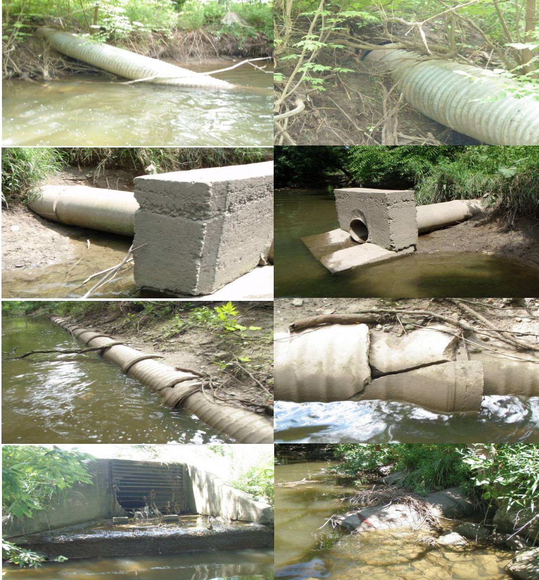
Figure 5.2 Outfalls Requiring Maintenance.
