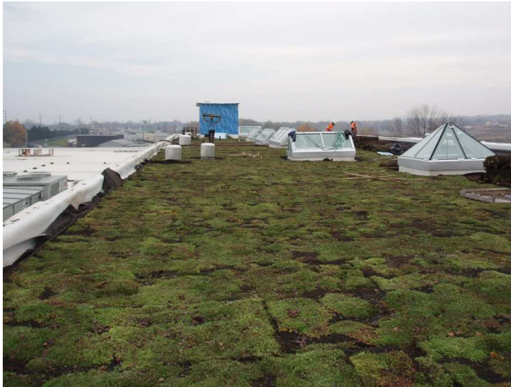
Figure 3.29 Example of a green roof being installed at GO Transit in Mississauga
