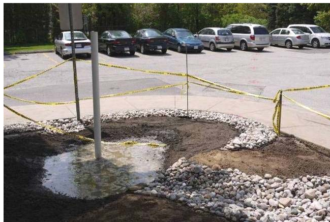
Water not properly draining into through the soil media
