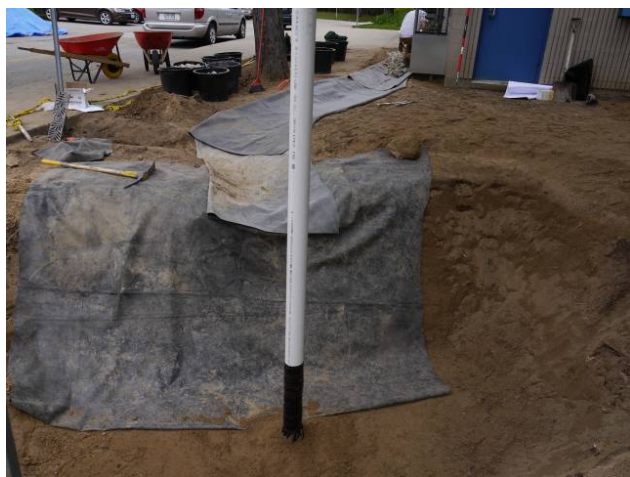
[Foreground]-observation well, [Background]-pond liner covering dry river bed and rear wall of the bioretention area
