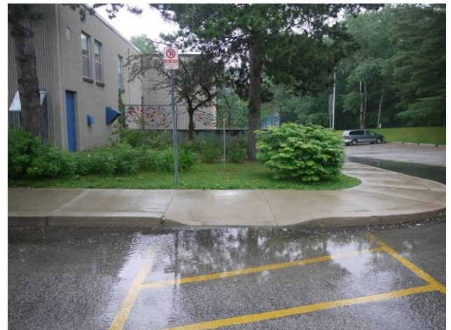
Nuisance ponding in pedestrian walkway
