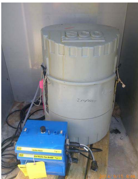
Figure 2: Monitoring setup showing the ISCO Area-Velocity Flow Module and an autosampler
